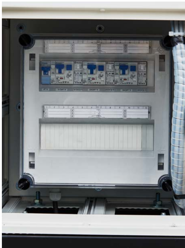
Technical compartment with power input
